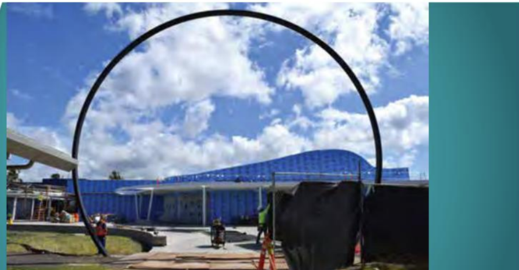
Constructors Hawaii completes expanded renovations at the Pacific Fleet Submarine Museum and Park. PHOTOS COURTESY CONSTRUCTORS HAWAII INC.
