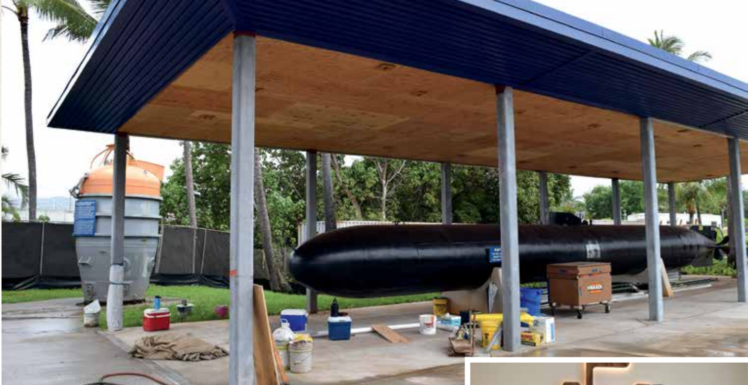
Constructors Hawaii's $13.3 million Pacific Fleet Submarine Museum project is targeting a June 2020 wrap.
