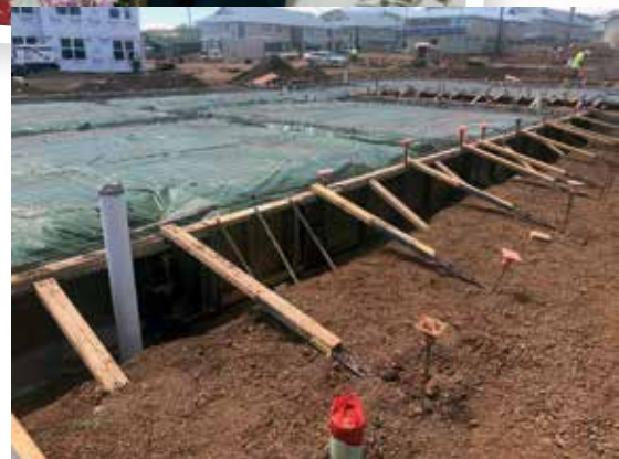
Koa'e Workforce Housing, a current Shioi project, will provide 134 units, 23 buildings and a community center. PHOTO COURTESY SHIOI CONSTRUCTION INC.
